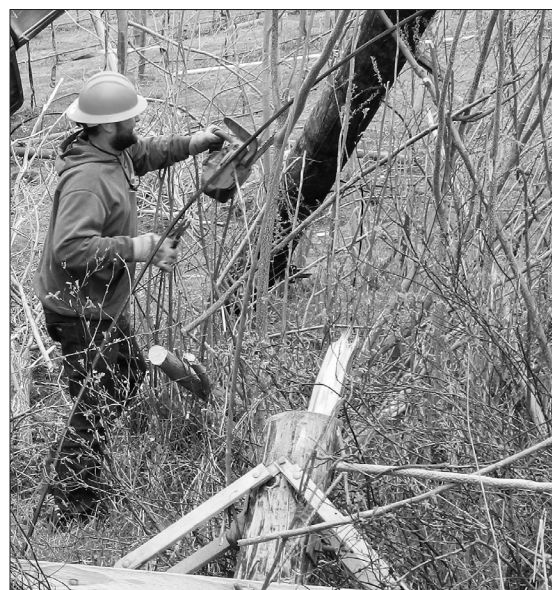
Bernie Predeek removes a broken pole from the site of a vehicle accident, to replace it with a new one and restore power.
