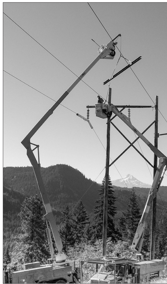
Repairs are made to the damaged structure on the Glenwood transmission line while the line remains energized. Lake Howard flies the cross-arm to Jeff Speelman and Todd Niva in the bucket.
